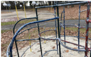
Underutilized space in Poplar Hall Park—outdated and children's playground in need of repair.
