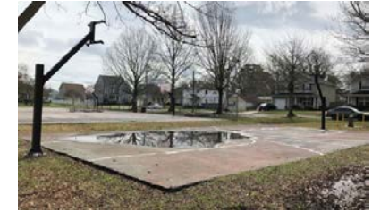
Ballentine Park Basketball court with poor drainage and missing backboard
